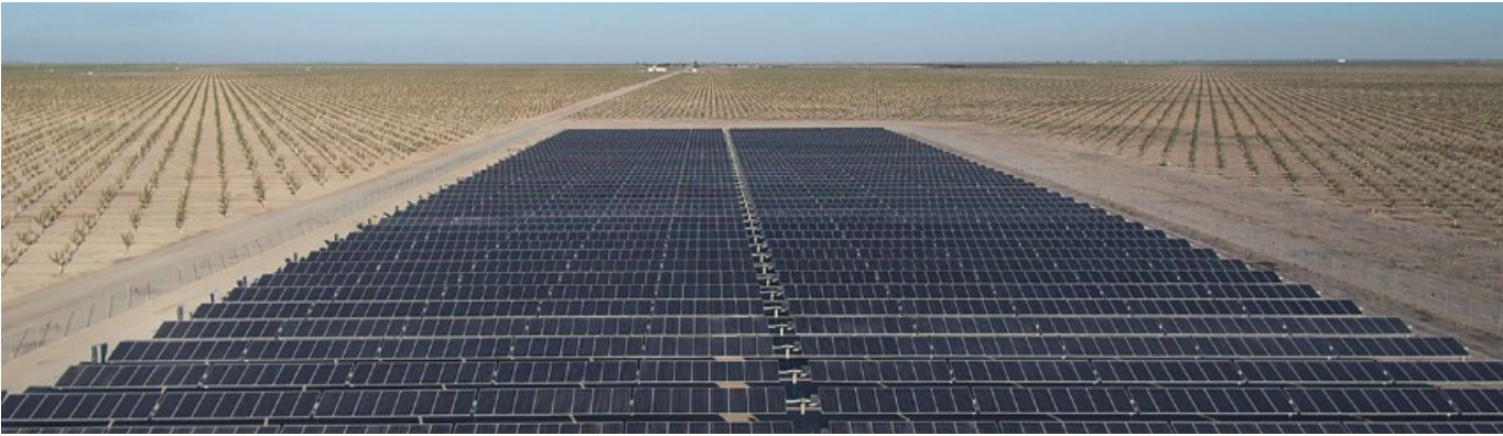
The new 3.9 MW solar array at our Triangle T Ranch provides 93 per cent of the electricity needed to operate the farm’s groundwater and irrigation wells and pumps. See the story on page 27 .
